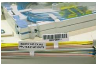
Fibre optic cable markers
