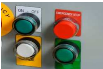
Control panel labels
