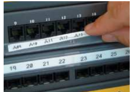
Punch block & patch panel labels
