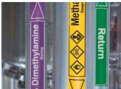
Pipe & valve marking
