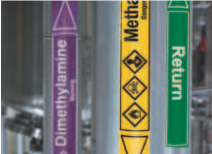
Pipe & valve marking
