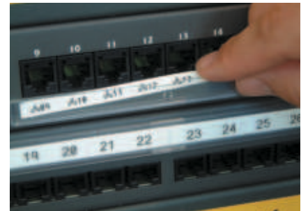
Punch block & patch panel labels
