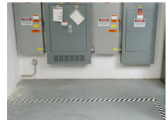
6. Colour-code areas in front of electrical panels.
