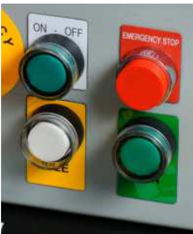
Control panel labels
